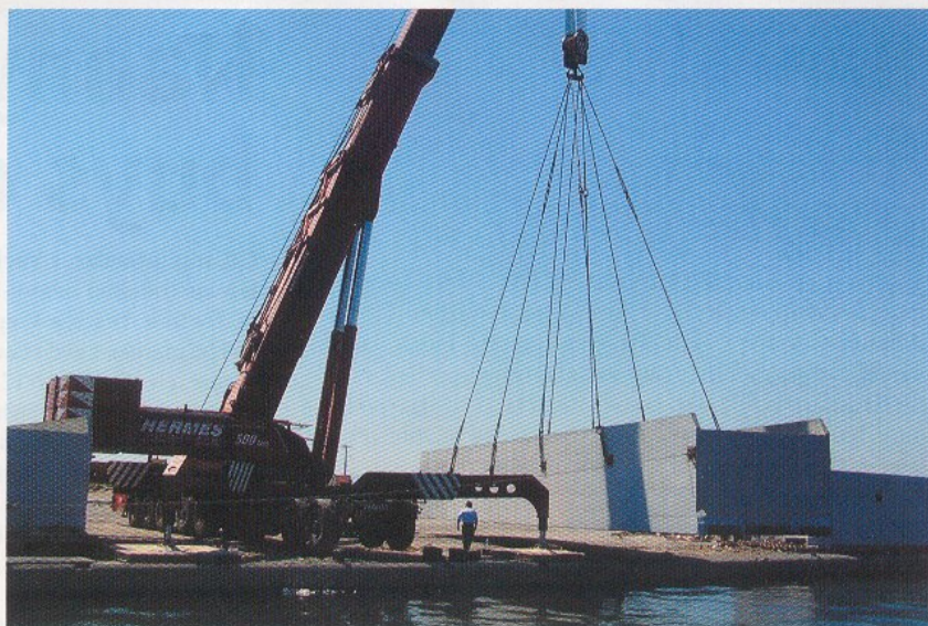
Lifting a breakwater unit for installation at the Olympic Marina of Faliro.
